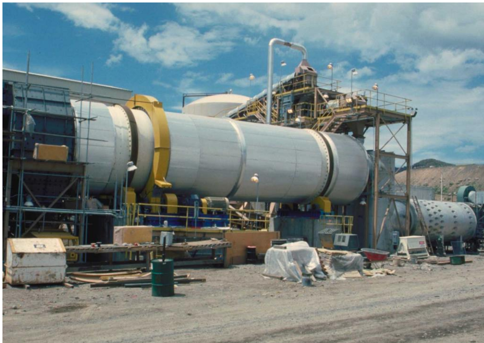
Image 2: Illustrative example of a conventional rotary kiln thermal dryer
