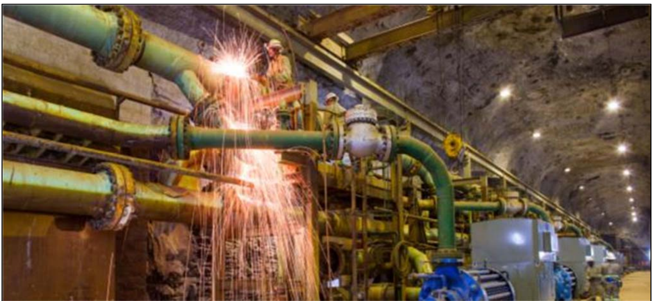
Figure 5: Welding at the Kipushi Mine's Shaft 5 pumping station in preparation for a resumption of production.
