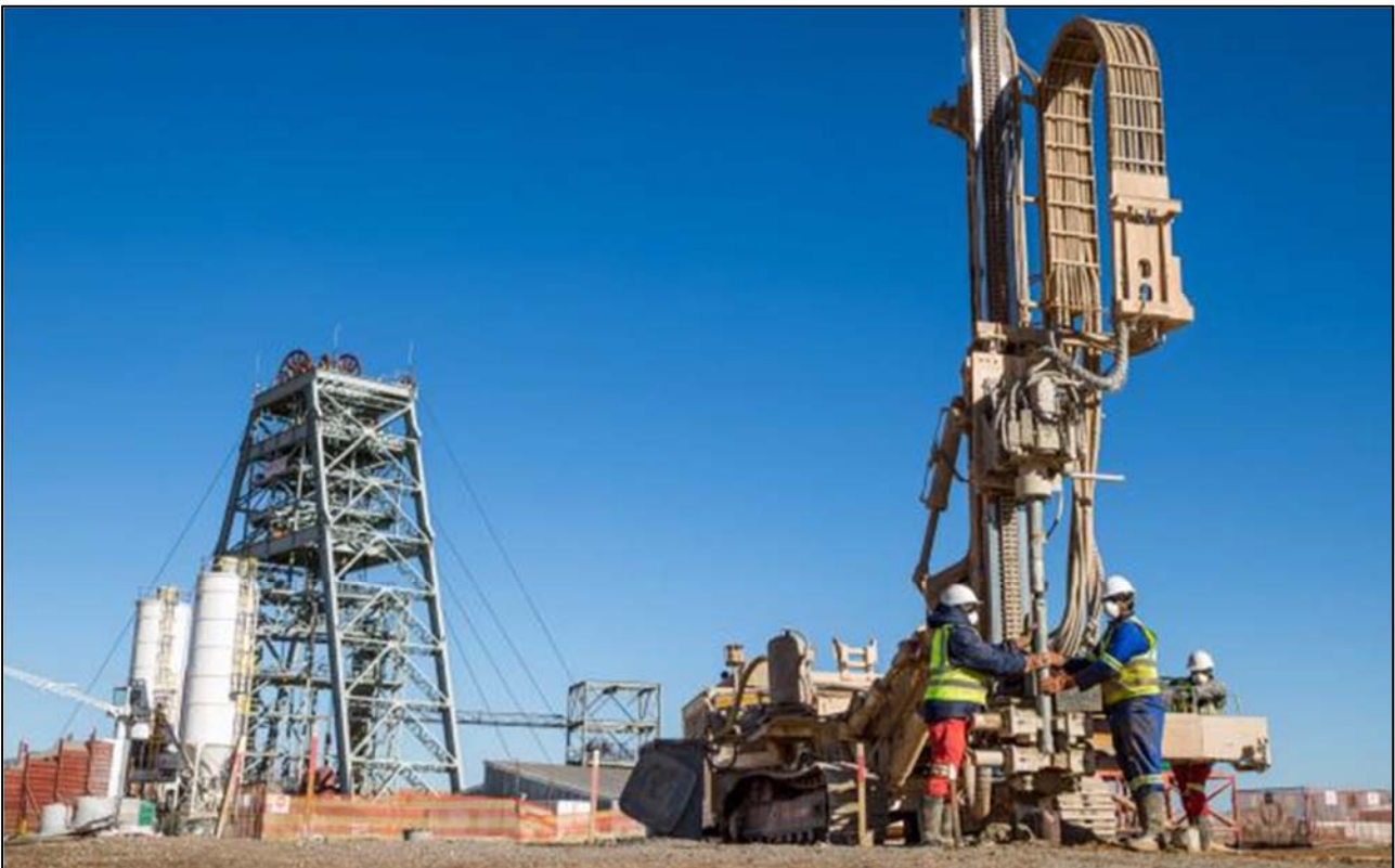
Figure 2: Drill-rig crew members during early-works surface construction at Shaft 2, located approximately 100 metres northeast of Shaft 1.
